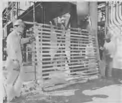
Workmen here show how the piping is prefabricated on racks at ground level. Note how swivel clamps are set in place ready for assembly.
